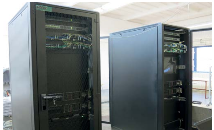
The heart of the system is Central Processing Station (CPS) that performs multilateration calculation, target, data and system management.
